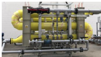
SEACLOR® Electrolyser EDF Dungeness Nuclear Power Plant, UK
